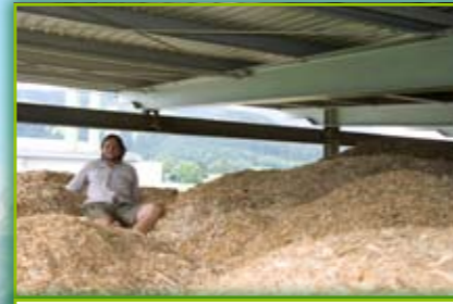
Obergailtaler biomass district heating plant
